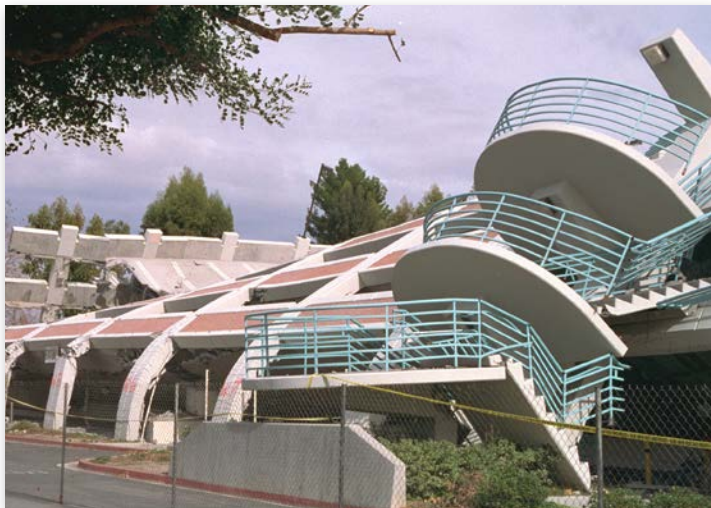
Concrete columns with inadequate confining reinforcement steel failed during the 1994 Northridge earthquake.
